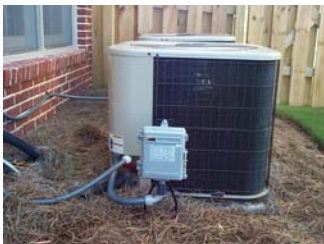
Installed load management switch
